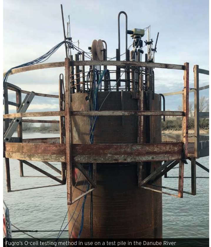
Fugro's O-cell testing method in use on a test pile in the Danube River
