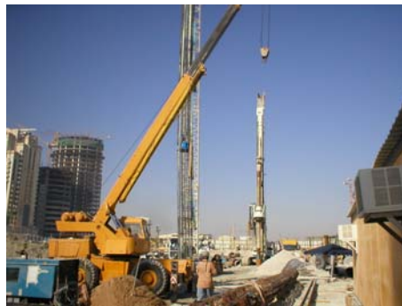
Pile cage installation on site in Doha, where many exciting projects are under construction
