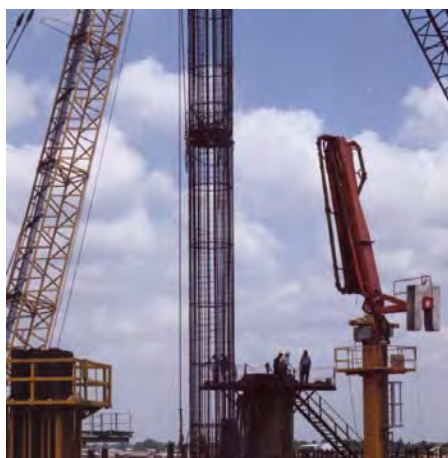
Test shafts/piles from 4.5-107 m have been successfully installed. Precast piles as long as 40 m have been driven and tested with the O-Cell.
