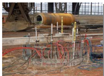
Test in progress (diaphragm wall grab and tunneling machine in the background)
