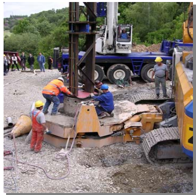
Installation of the O-cells on the steel carrying frame into the pile bore
