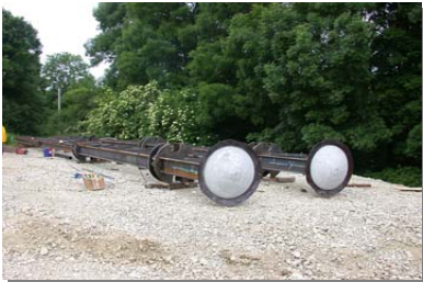
Installation of O-cells and pressure cell on the bottom of the carrying frame
