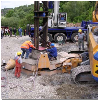
Installation of the O-cells on the steel carrying frame into the pile bore
