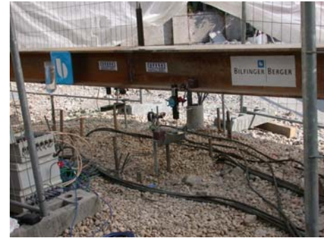
Bi-directional test in progress. The steel beam shown in the picture is being used as a reference frame from which pile top movement was measured.
