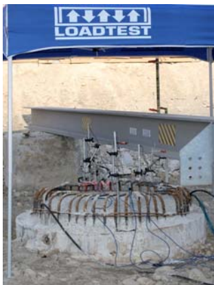
Pile head test arrangement showing reference beam during O-cell bi-directional loading in progress.
