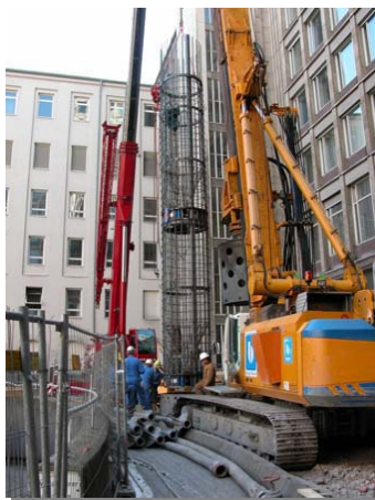
Installation of the bottom section of reinforcing cage with both O-cell arrangements
