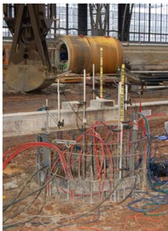
Test in progress (diaphragm wall grab and tunneling machine in the background)
