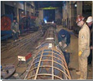
Pile cage assembly built in a workshop and later transported to site for installation
