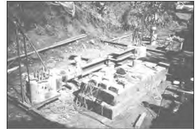
Figure 1 - Datalogger system used to monitor instrumentation during a lateral load test
