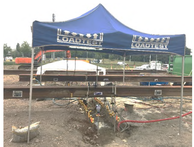
Top of barrette instrumentation setup. Note the reference beams across each of the O-Cell® tests
